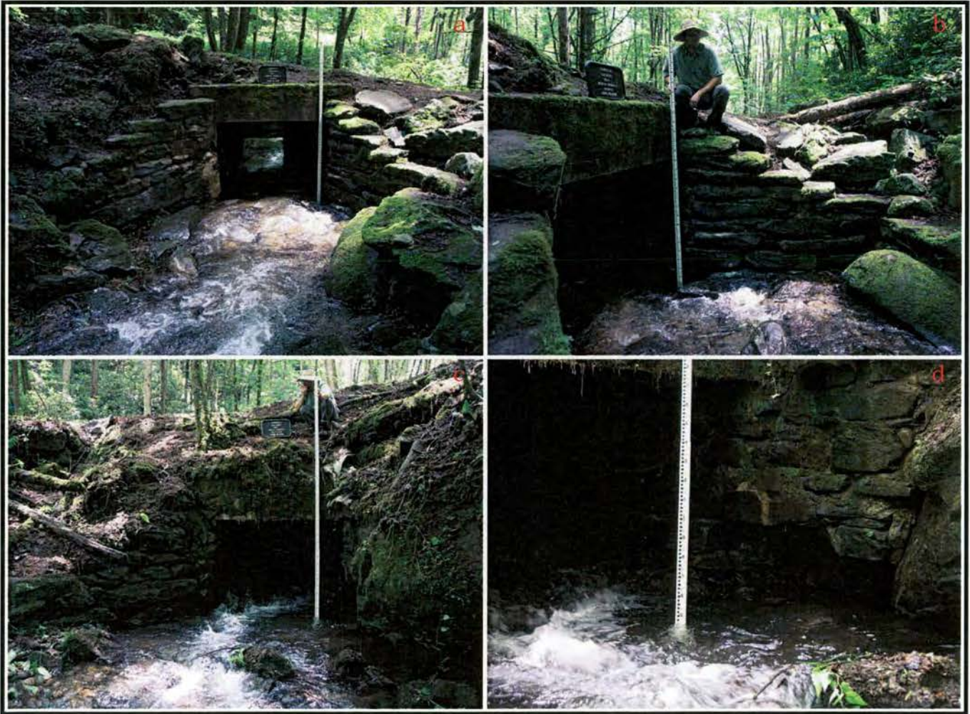
Figure 8. Overview photographs of Culvert No.1 on Shope Fork: a) intake and wing walls, view to northeast; b) close-up of southeast wing wall of intake, view to east; c) outflow and wing walls, view to south; d) loss of stones at base of west wing wall of outflow, view to southwest.
