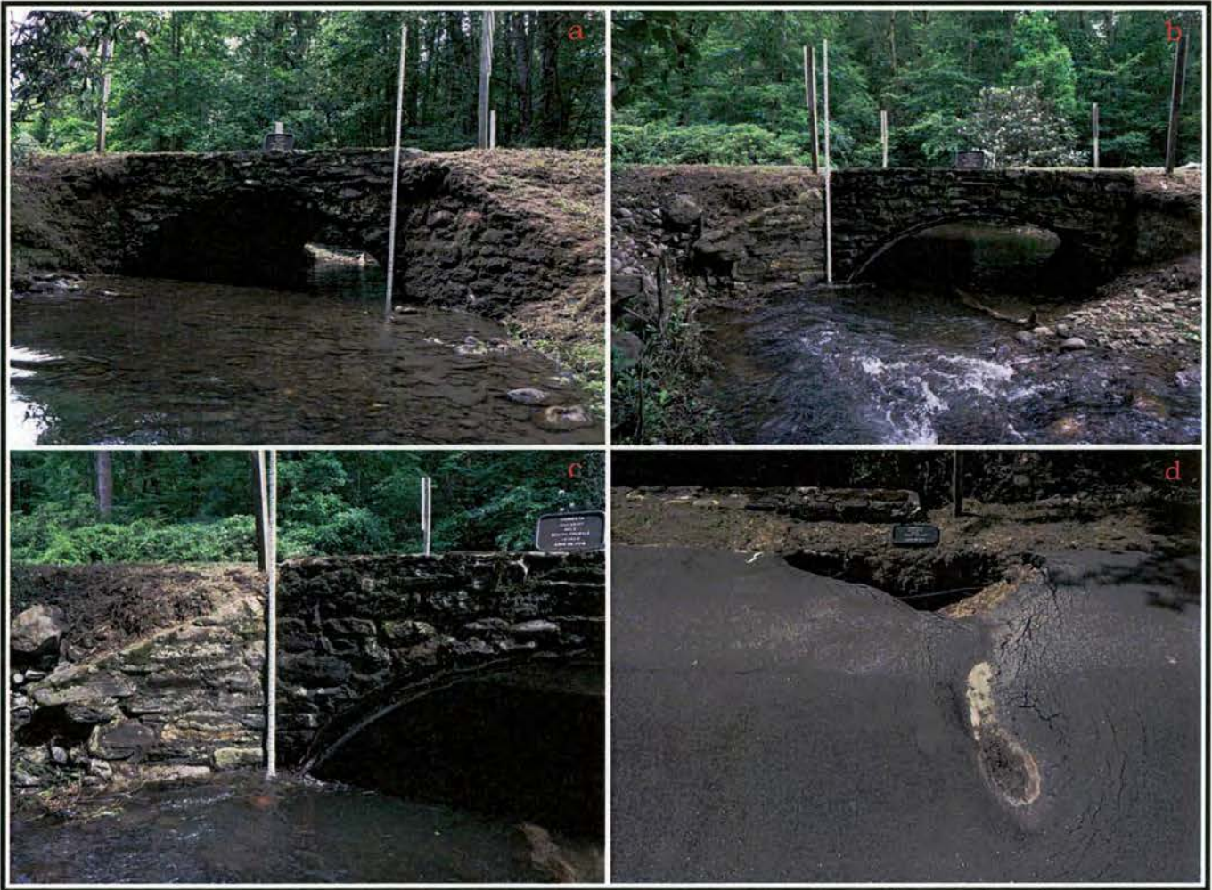
Figure 9. Overview photographs of Bridge No. 1 near confluence of Shope Fork and Ball Creek: a) outflow and wing walls, view to north; b) headwall and wing walls, view to south; c) damaged northeast wing wall and CSP liner, view to southeast; d) Forest Road 83 failure, view to north.
